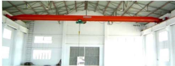
LH electric hoist double girder bridge crane
